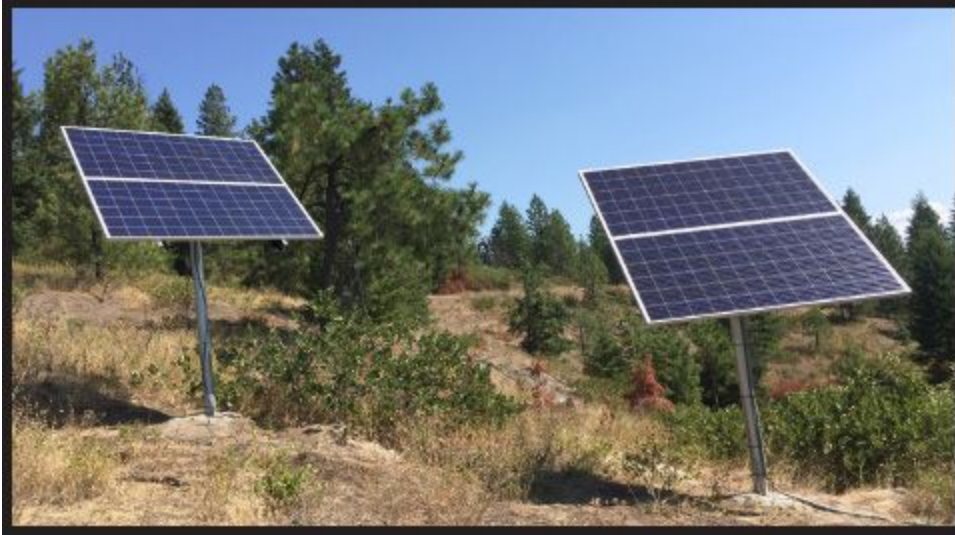
Moveable solar panels
