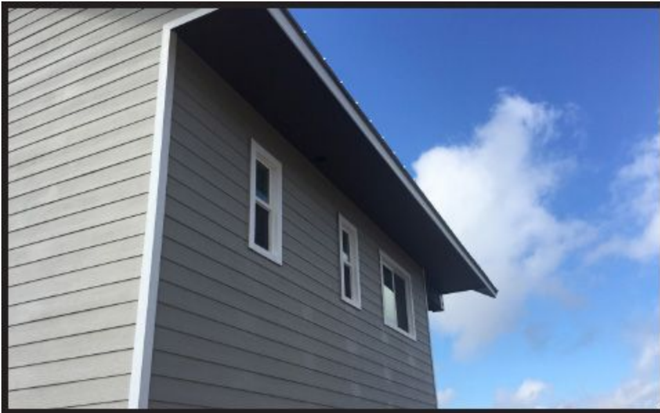
Fire-resistant siding on my house
