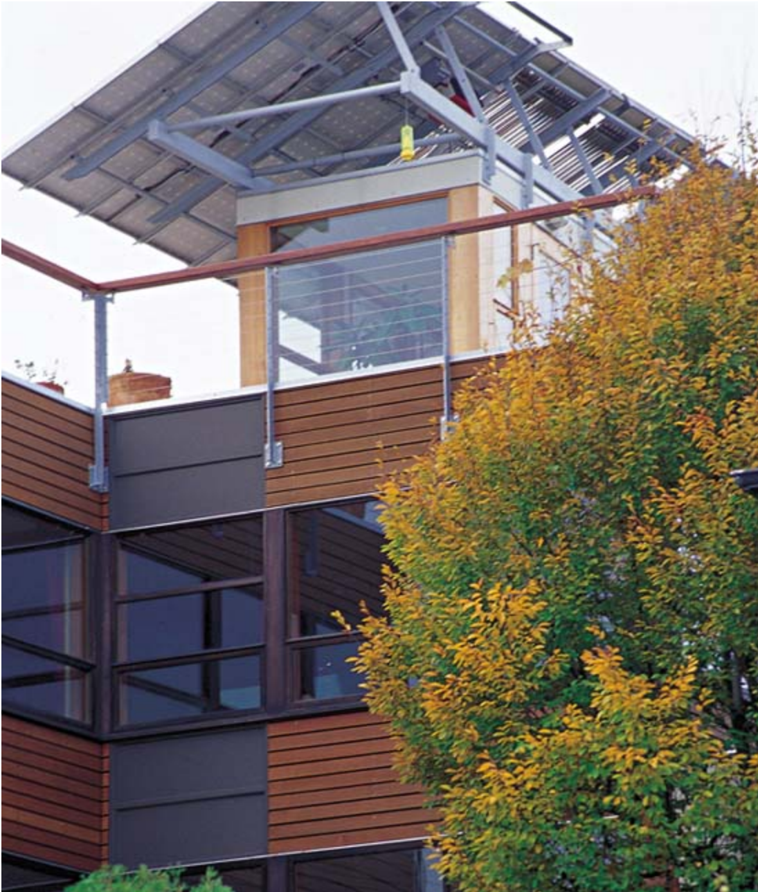
The PV array and solar hot-water heater are simply mounted to a steel substructure angled for optimum solar collection.
