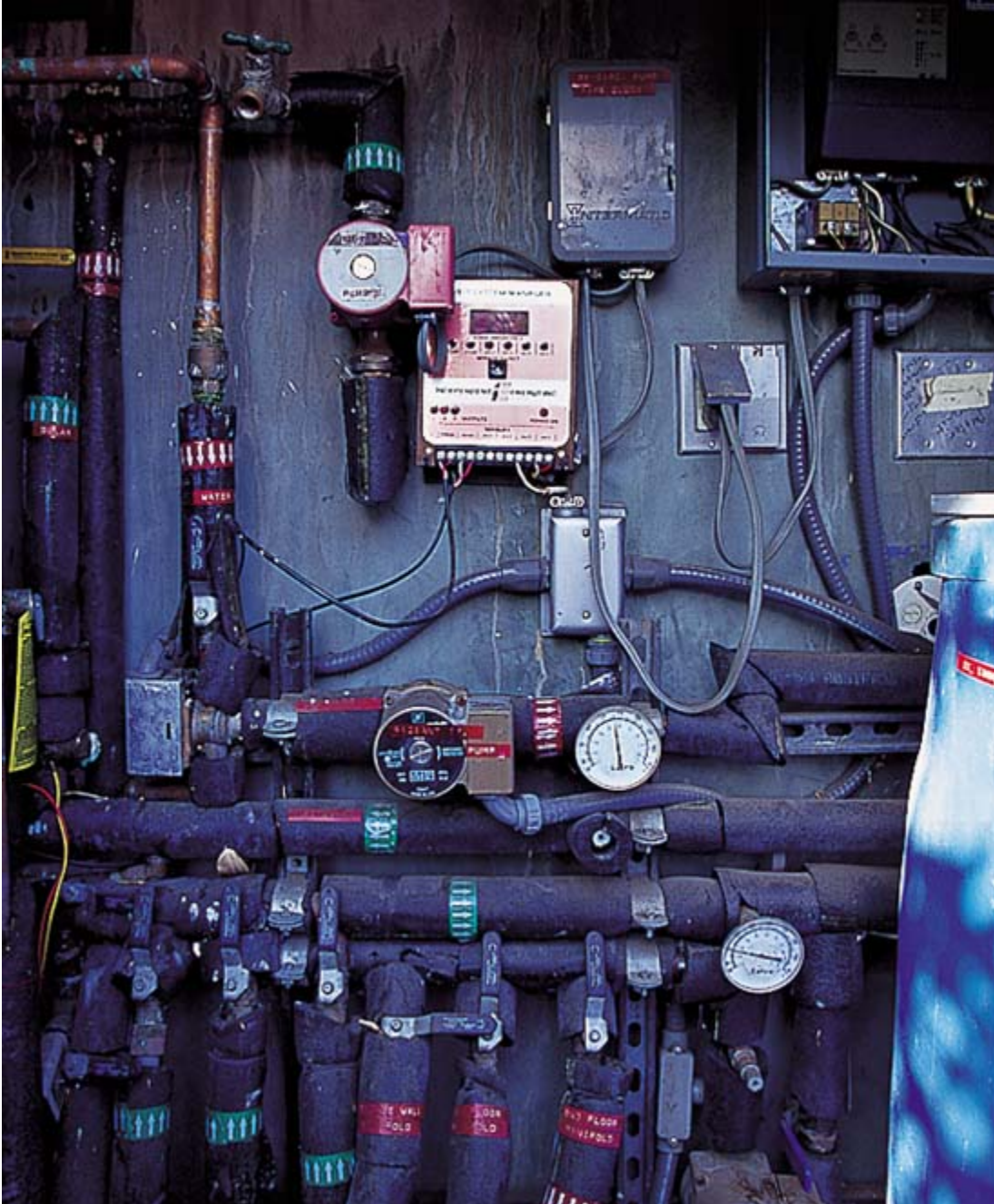
Most mechanical rooms look unapproachable to a lay person. This system includes a PV inverter added to a pre-existing mechanical system. While it may appear complicated, such an addition is quite simple for most electricians.
