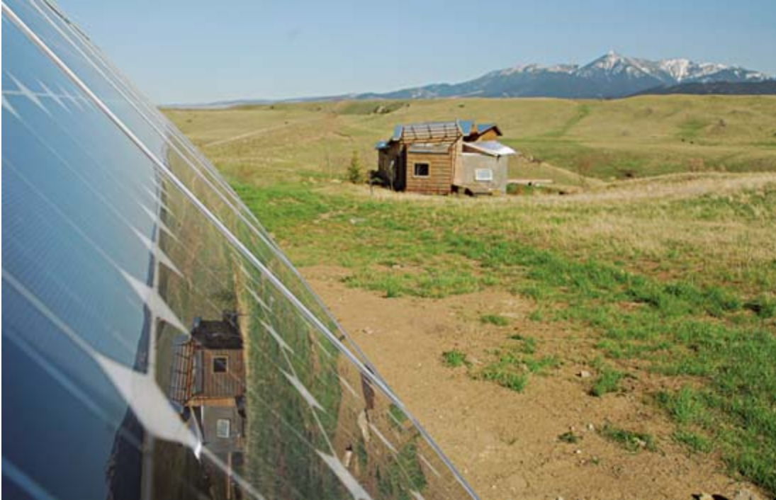
A 1,800-kWh PV array, custom mounted to the shop, provides almost 50 percent of the electrical requirements for the house.
