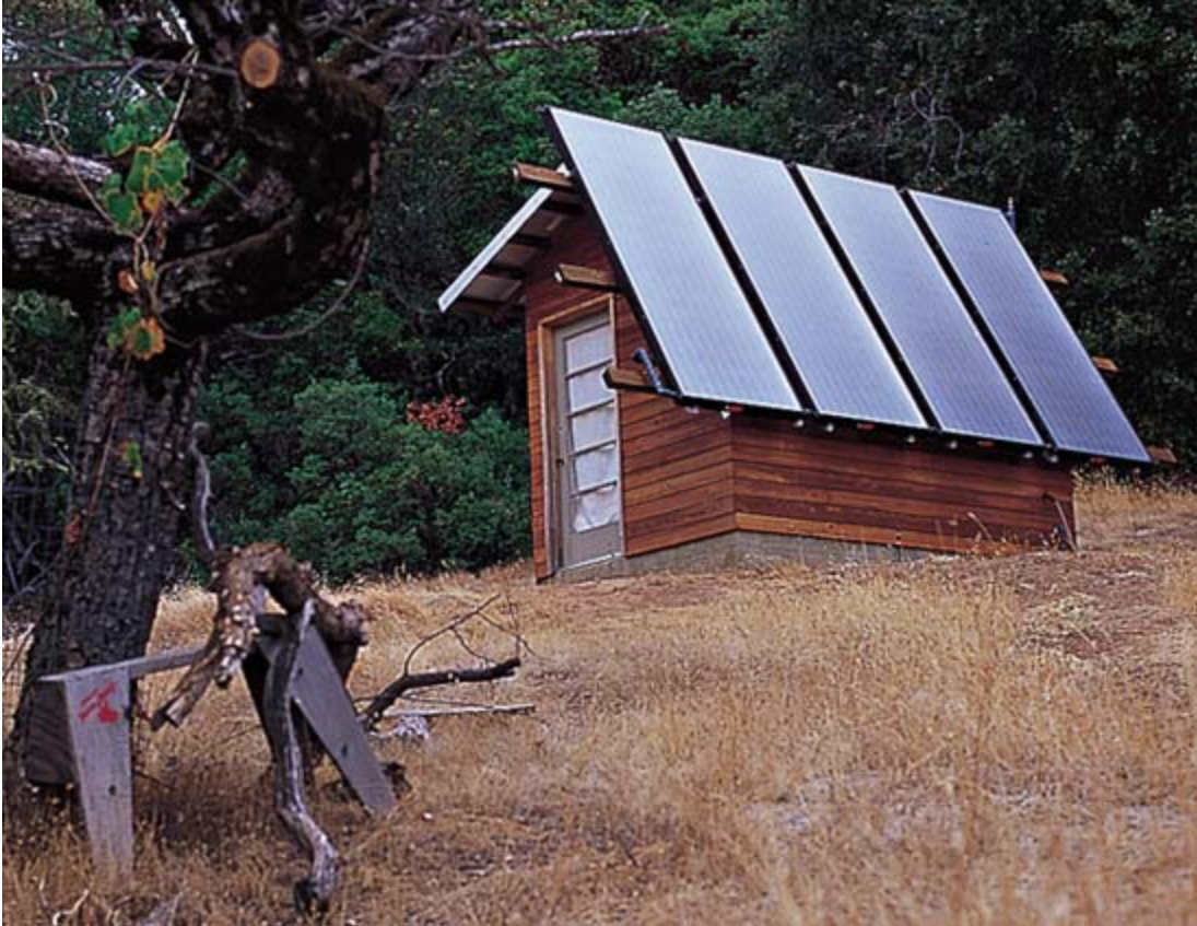
Solar hot-water panels mounted to the adjacent shed provide domestic hot water and heat for the radiant floor system.
