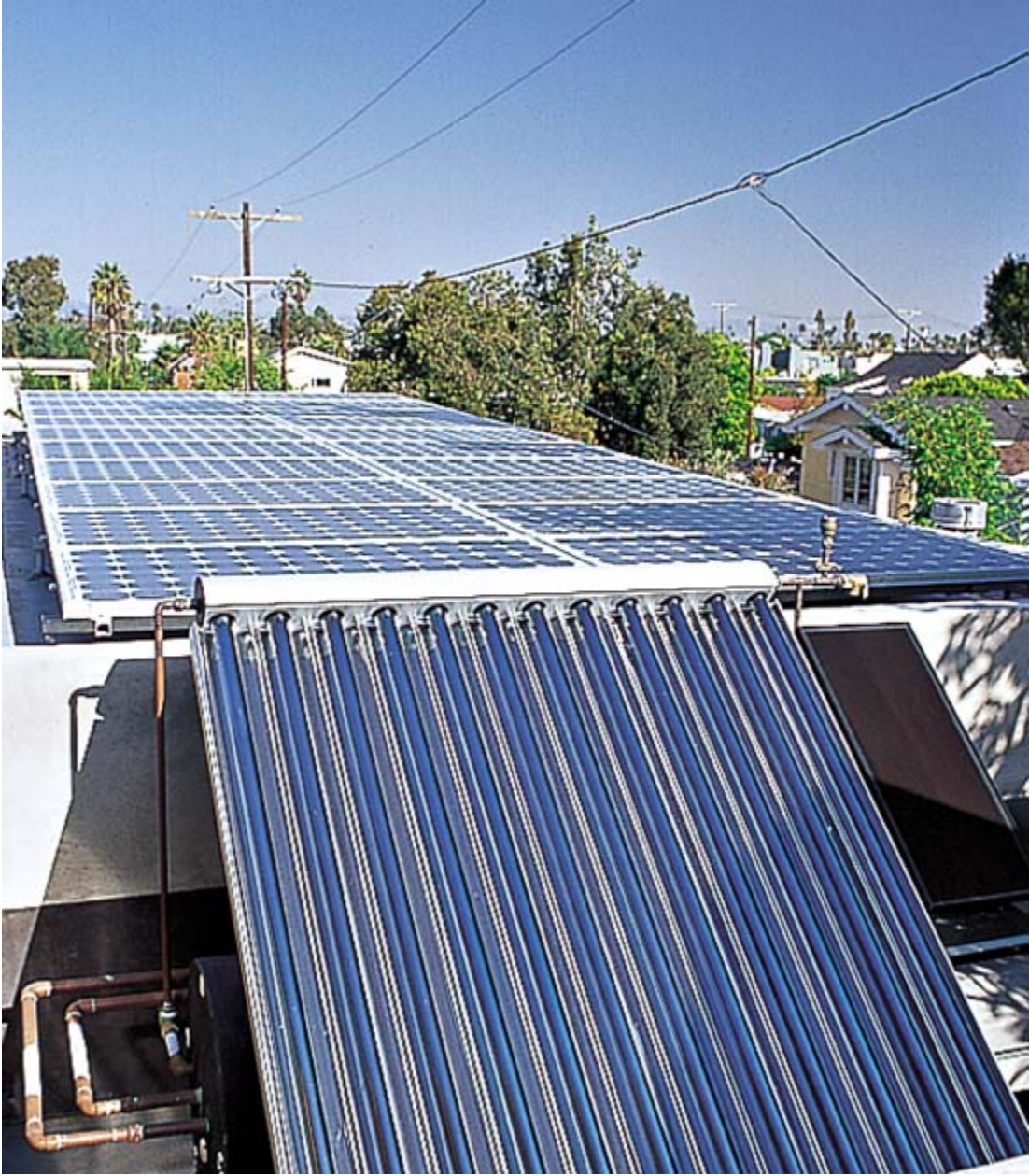
Solar hot-water heaters share rooftop space with PV panels.
