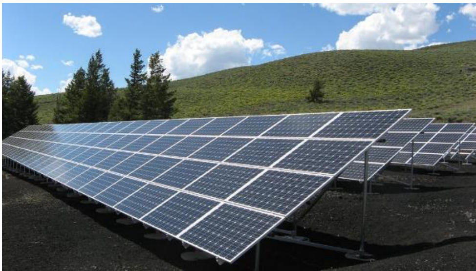
Solar panels in a field. Often times done for shared or community solar energy resources.
