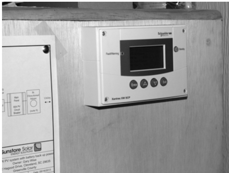
SOLAR CHARGE METER
