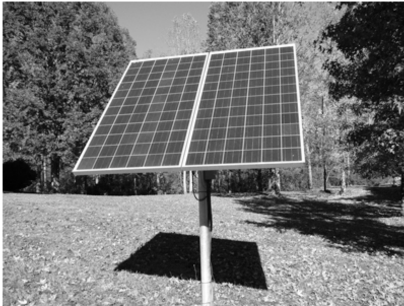
“PHASE TWO” SOLAR ARRAY
