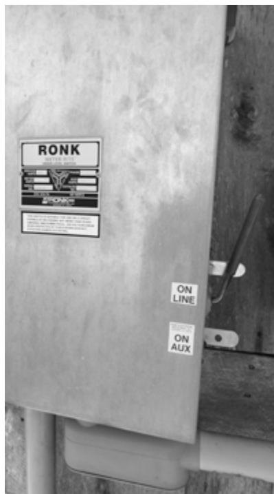
MANUAL GRID DISCONNECT
